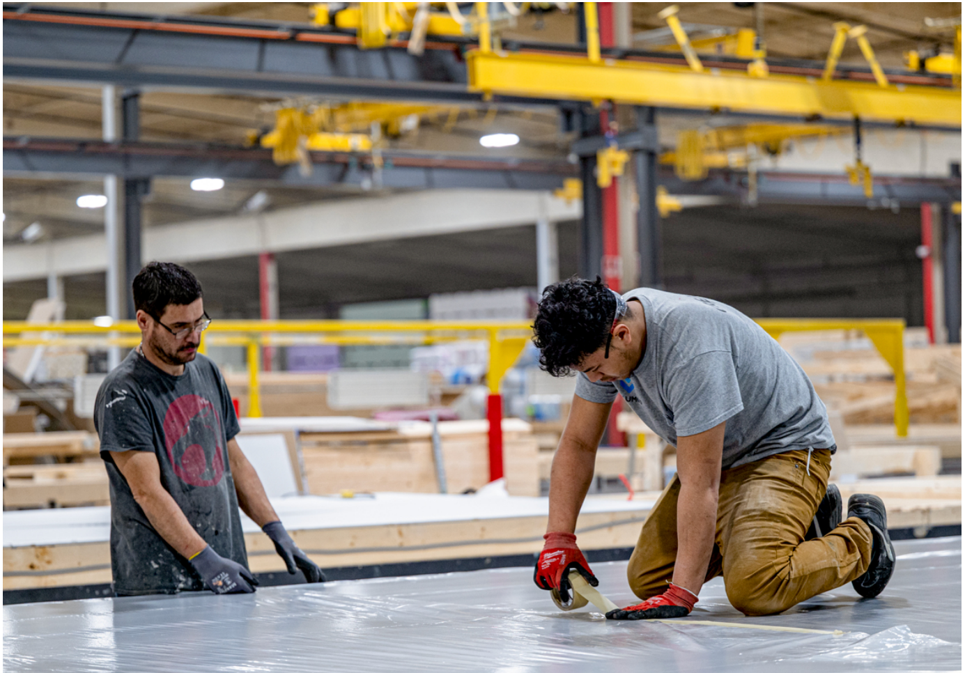
Volumod workers build housing units in an assembly-line fashion at the P30 coworking space at 3039 N. Post Road. (IBJ photo/Mickey Shuey)
