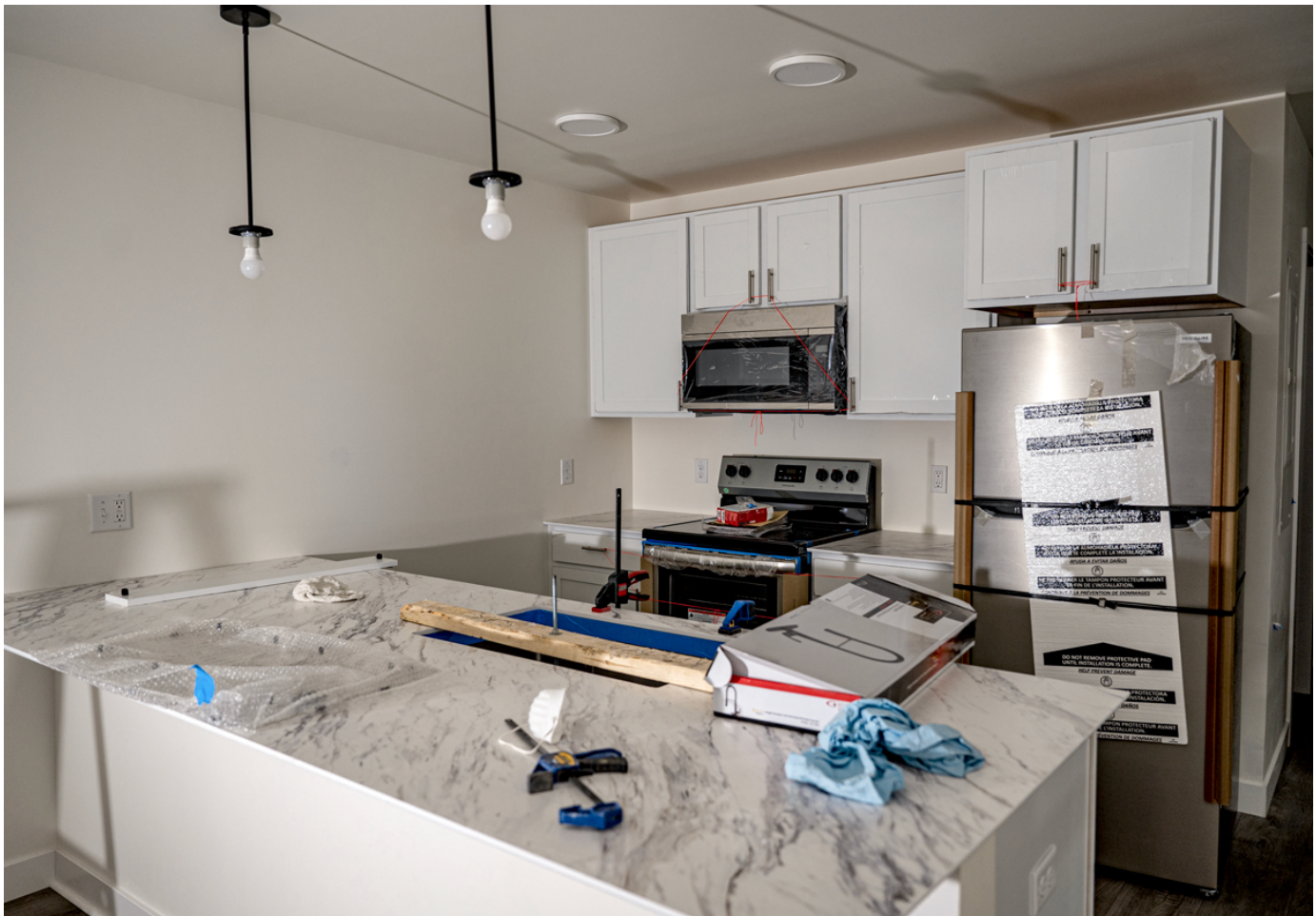
Volumod's pre-built modular units come with the kitchen appliances already installed. (IBJ photo/ Mickey Shuey)
